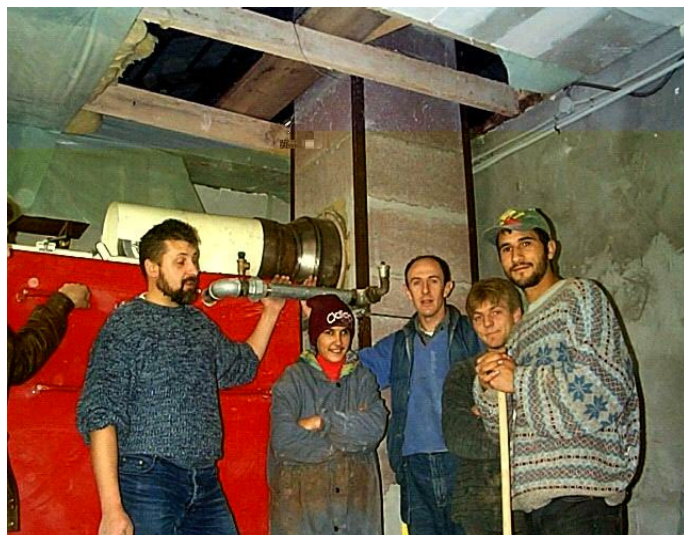
Chimney finally in place! Mr.Horvath, left, looked up oven: Aranka,Andrei,Florin, Remusn near by.
